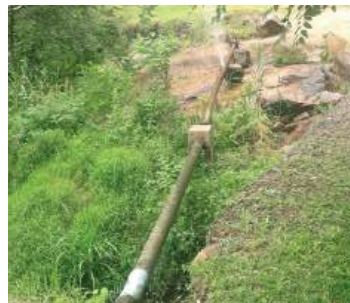
Current state of affairs on the pipeline of the Lichenya Water Supply Scheme.
