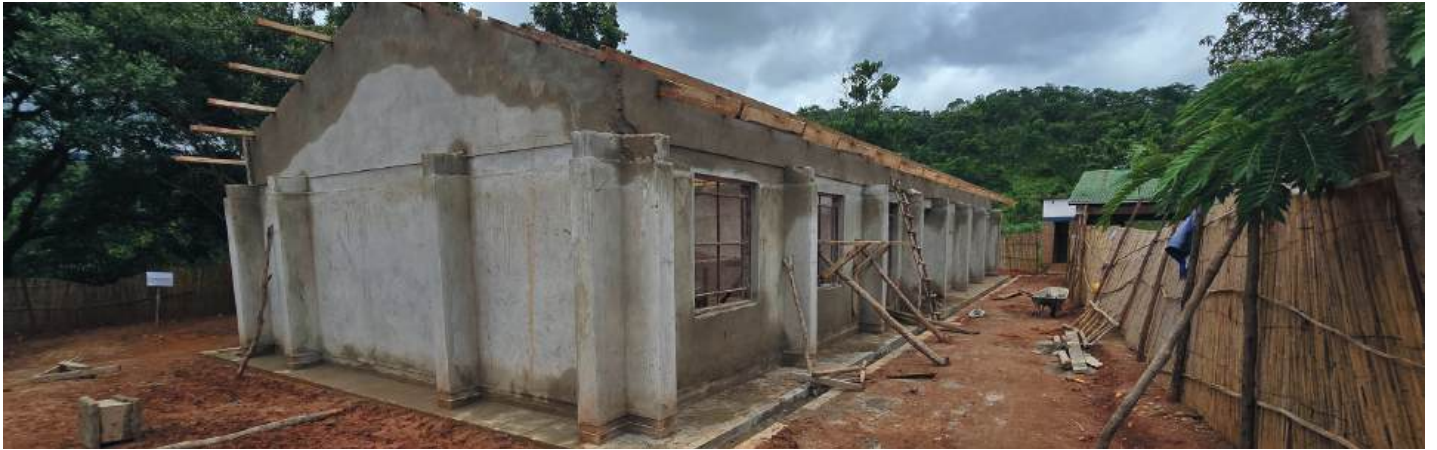
Progress of works at Mkuluzi Primary School in Nkhata Bay. Picture by Yvonne Sundu.
