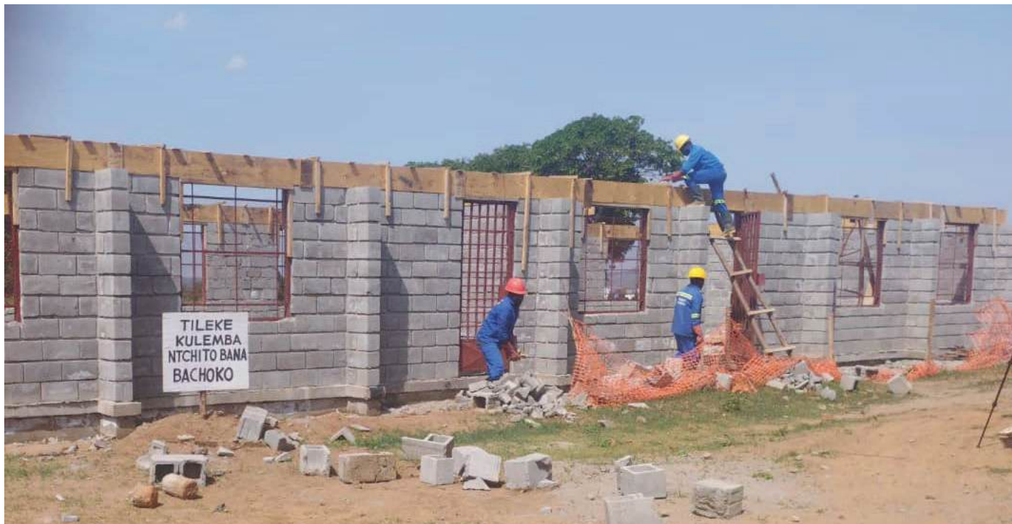
Progress of the school block at Kabowoza Primary School in Mzimba. Picture by Joel Phiri.
