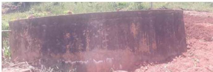
An old storage tank at the Chididi Water Supply Scheme.
