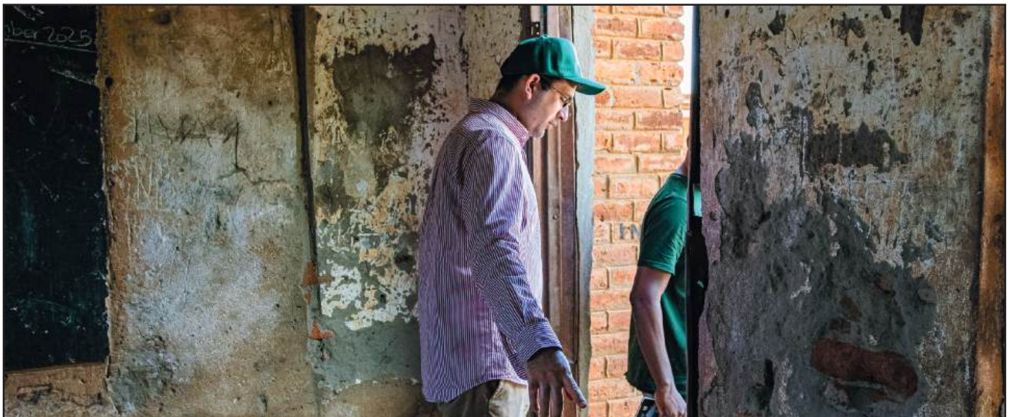
The dilapidated state of the inside of a classroom at Mseru Primary School. Picture by Yvonne Sundu.
