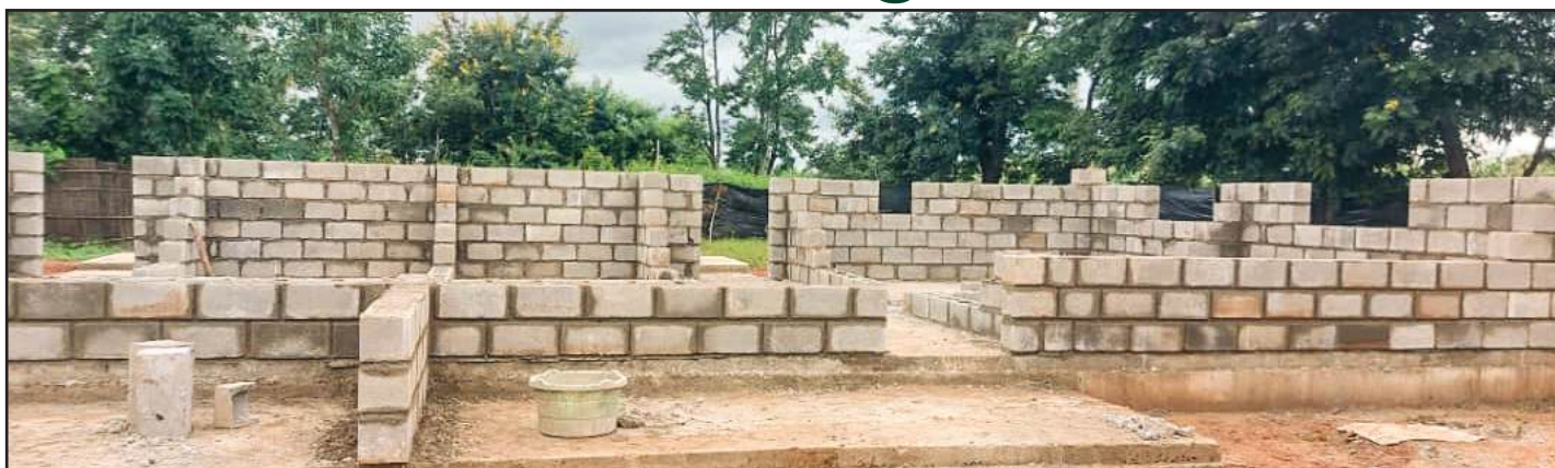
Progress of the staff house at Mseru Primary School in Lilongwe. Pictures by Yvonne Sundu.
