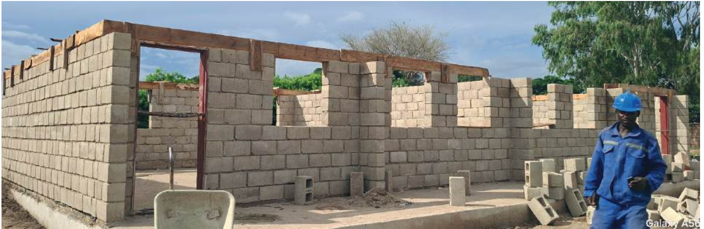
Ring beam formwork installation at Karonga Guardian Shelter. Picture by George Mponda.
